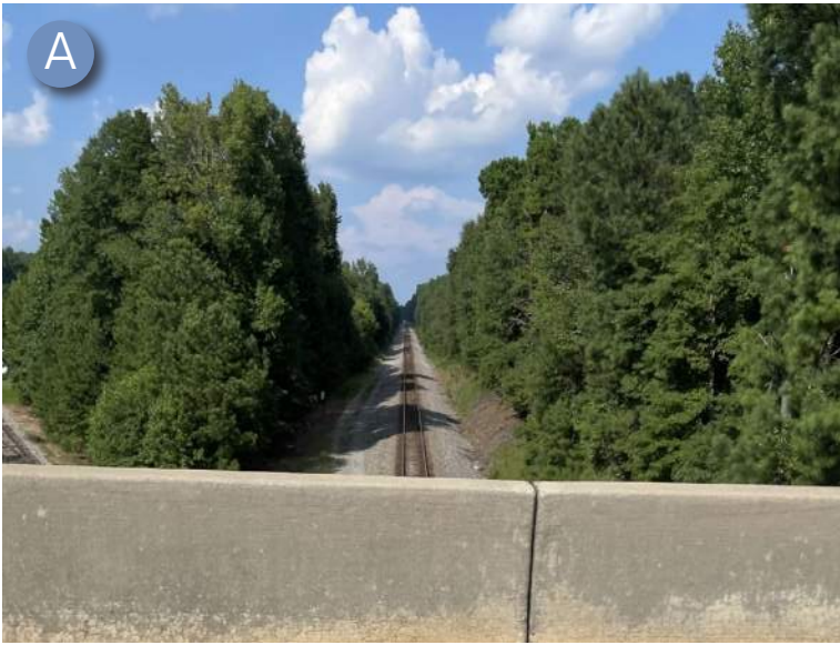
The trail could cross beneath HF Reed Industrial Parkway using the railroad underpass.
