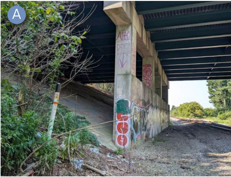
The trail could be raised into the slope on the other side of the bridge piers if the railroad gives permission to use their right of way.
